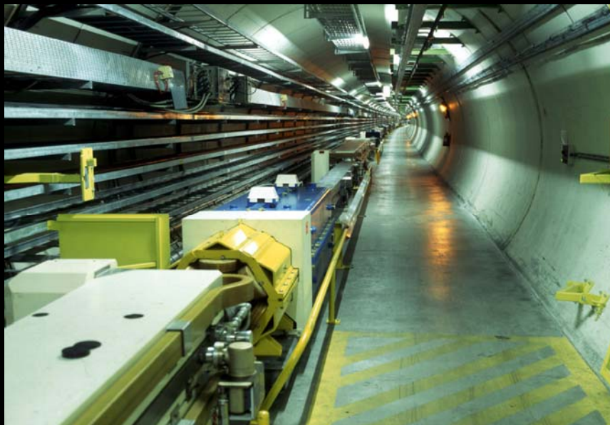
In Tunnel 150m underground, 27km ring of Magnets Keep electron in Circular Orbit
